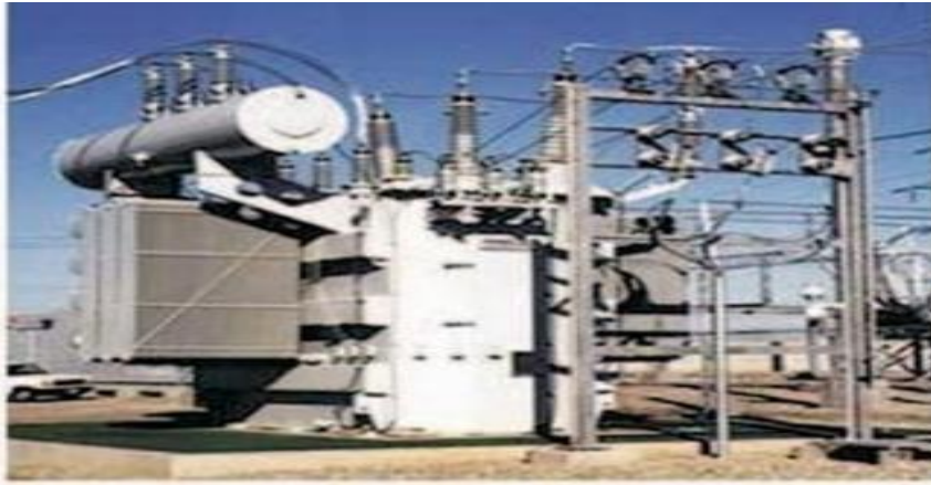
Figure View of a Transformer
